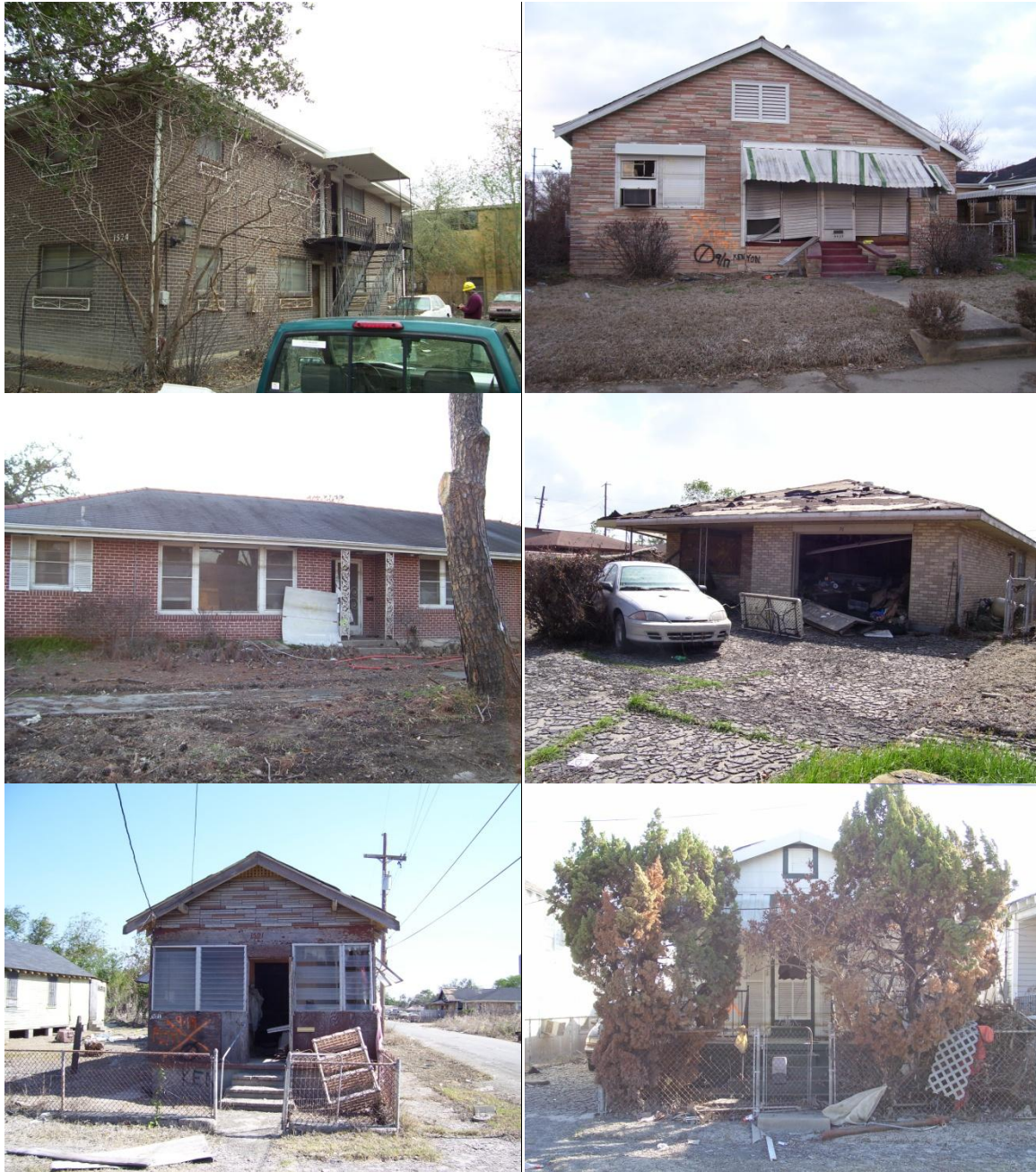
Figure 6.10: Sample of flooded residences from which deceased victims were recovered (Photos by Author).
